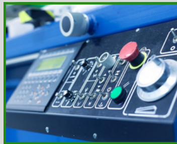
Industrial Machine Control Panels
